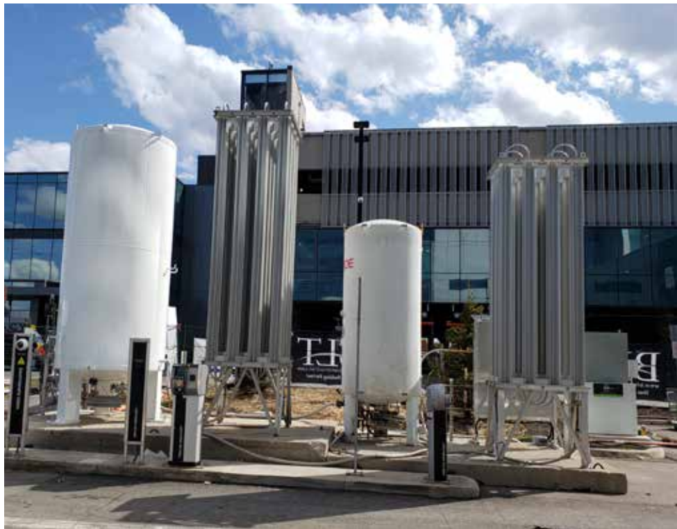
▲ A bulk oxygen system is being installed to supply a pandemic response unit at an Ontario hospital.
